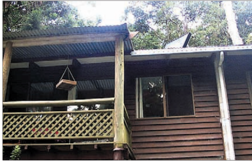
FRESH APPROACH ... Solitude retreat at Natural Bridge has installed SolarVenti to keep fresh air in its cabins.
