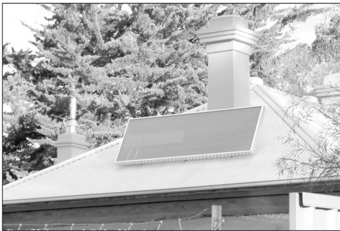
A roof-mounted Solarventi unit.
